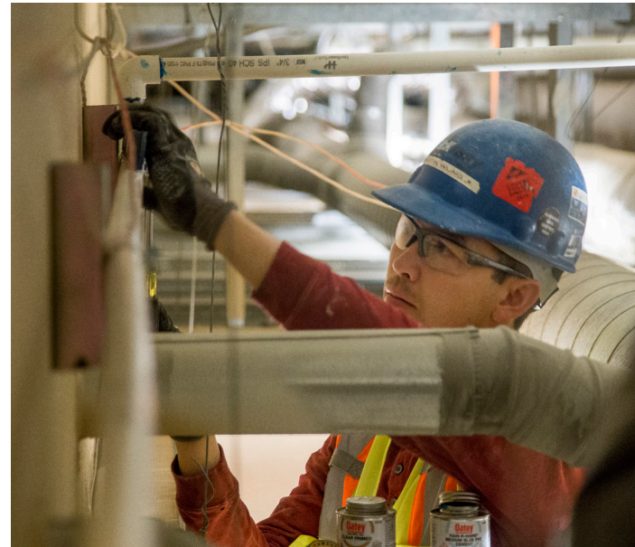
Renton, WA — PVC condensate line installation at a 2% (1/4-inch per foot) slope utilizing conventional hangars and unistrut supports.
